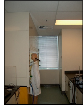
An example of the worst type of grill and bad location
