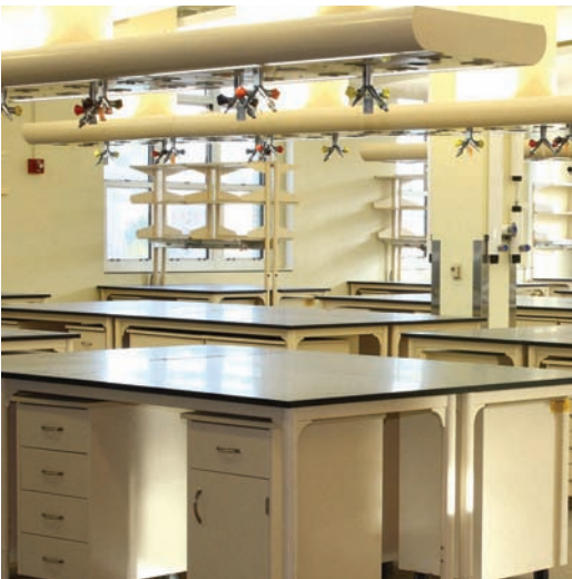
Custom designed configurations to accommodate all overhead service requirements.
